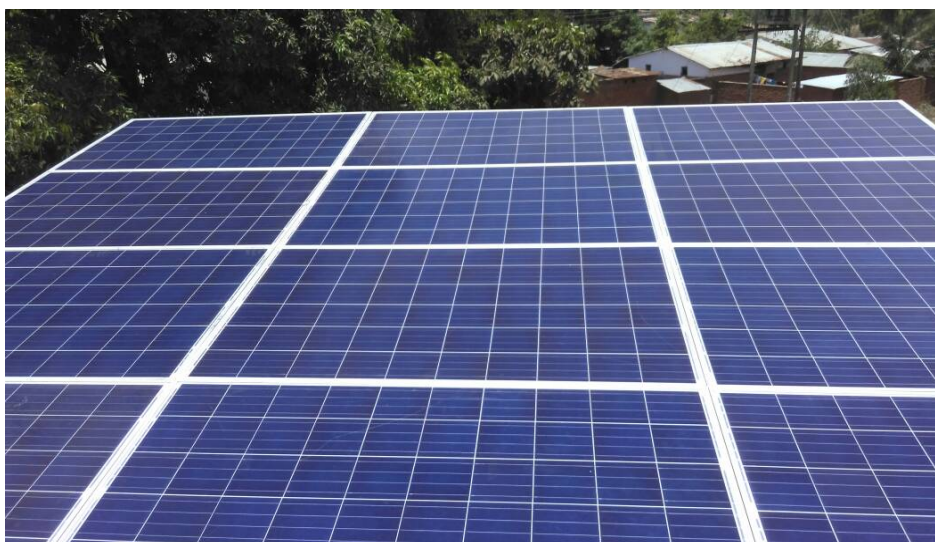
Figure 5.: Solar powered MBG milk cooling facility
